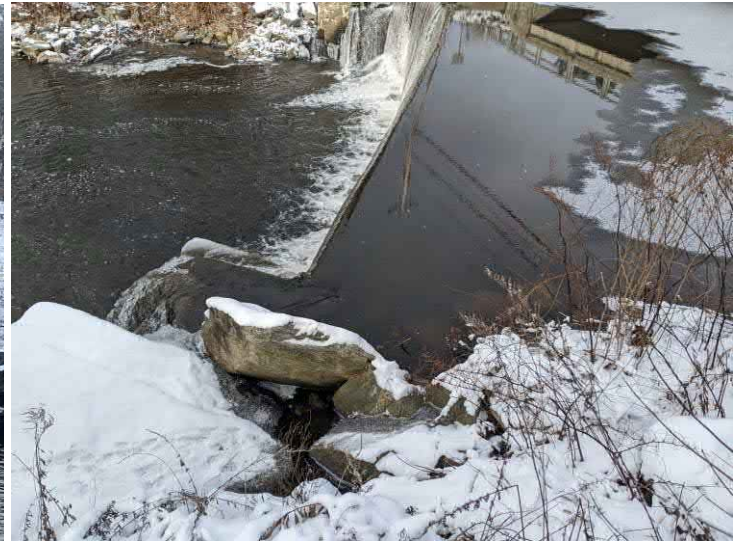
November 2021 – Flow through left abutment
